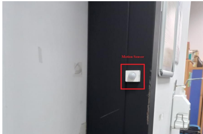
Figure 5. Motion sensor 1 in Room 1
